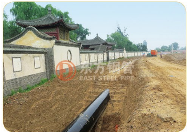
The Water Supply Project for the Beijing Yanqi Lake International Convention and Exhibition Center of 2014 APEC Summit
